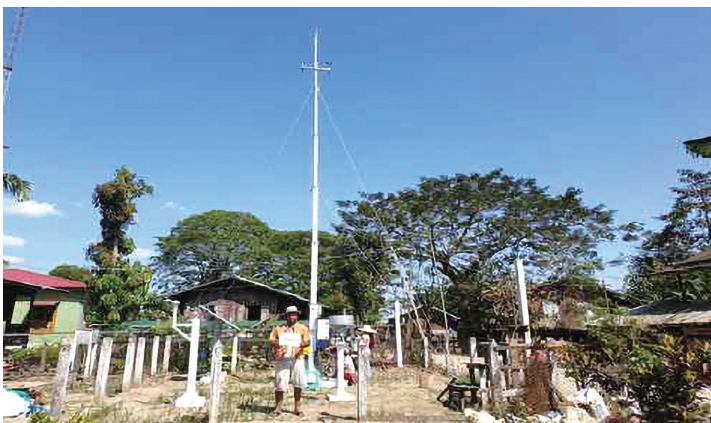
▲ AWS installation site in Homalin
